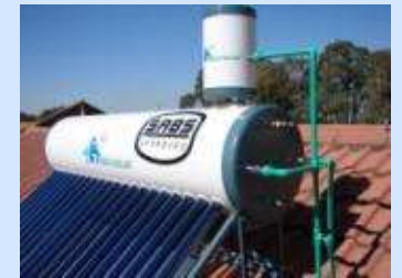
Solar hot water heaters
