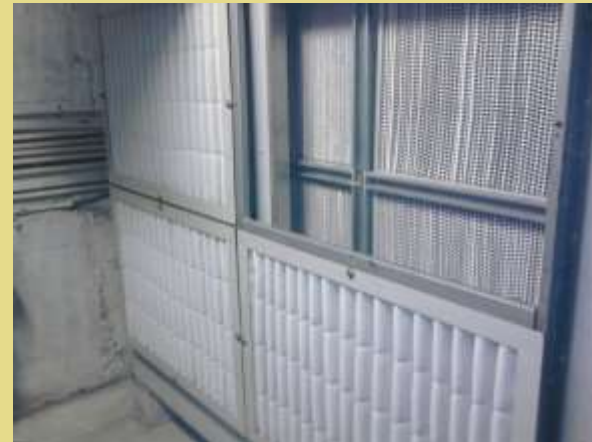
After retrofit with water washable G4 filter and air cleanable F7 filter
