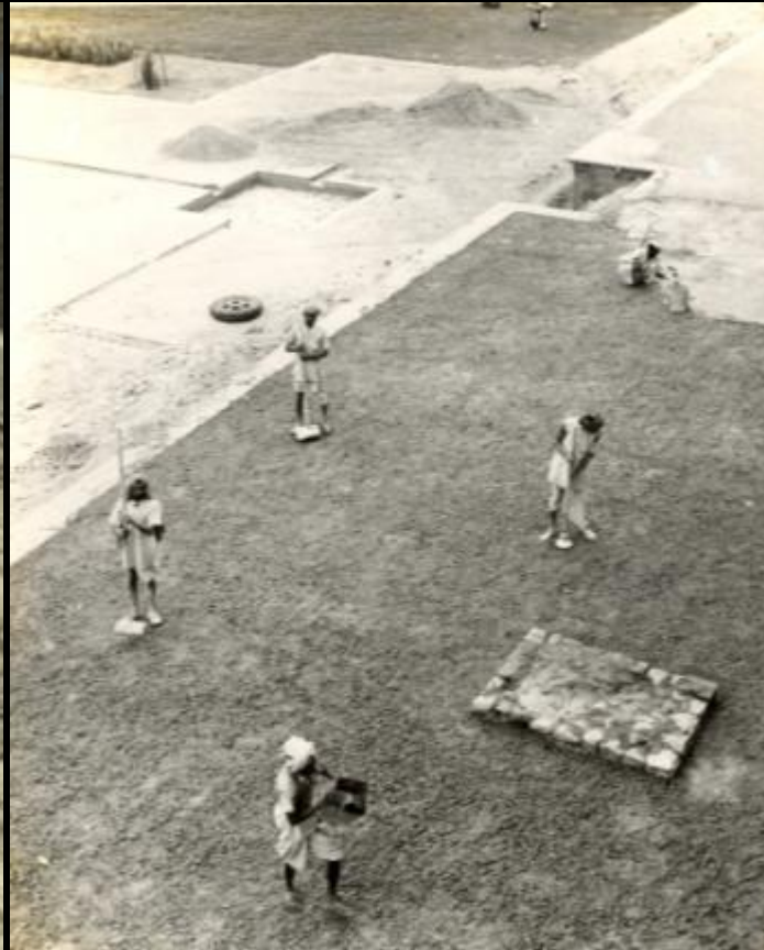
Concrete laid in 1950's
