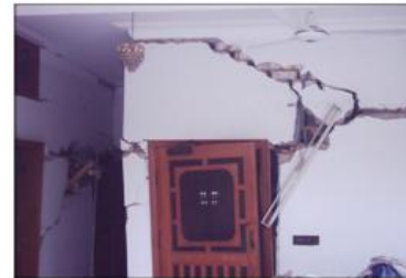
(a) Damaged unreinforced brick masonry wall in Muzaffarabad
