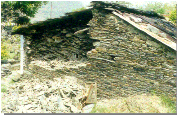
(b) Collapse of typical stone and slate wall with slate roof
