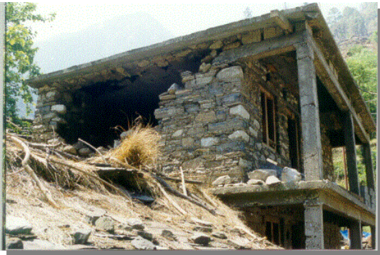
(a) Collapse of slate and stone masonry wall with poorly designed RCC construction
