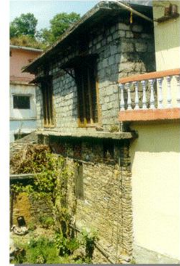
(b) Little Damaged concrete block masonry constructed over stone and slate masonry wall during Chamoli Earthquake
