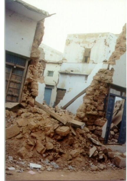
Damage to random rubble stone masonry at Anjar during Gujarat Earthquake 2001
